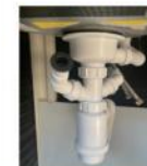
Wastewater discharge Dishwasher connection
